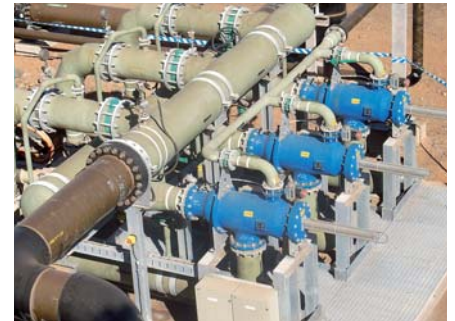
3 x 16" / DN 400 KAF Filter desalination
