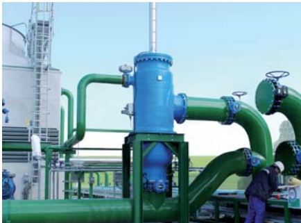
24" / DN 600 KAF Filter Bioethanol plant
